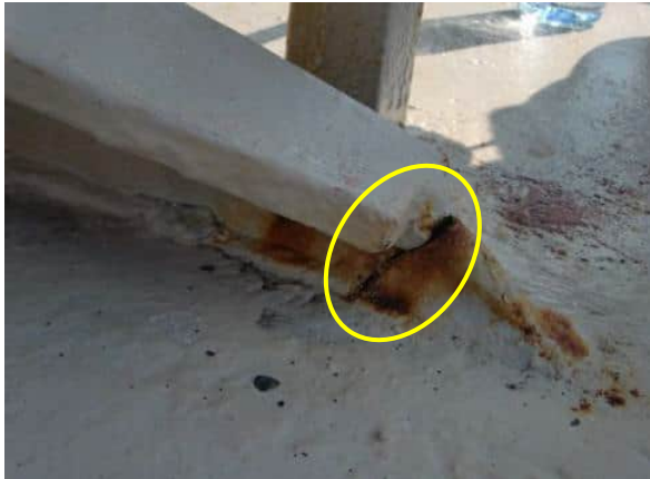
Cracked hatch coaming end bracket.
